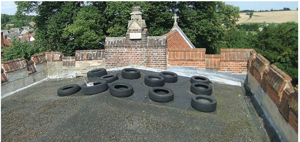
Nave roof prior to repairs at Wethersfield, St Mary Magdalene. © Ben Walmsley
