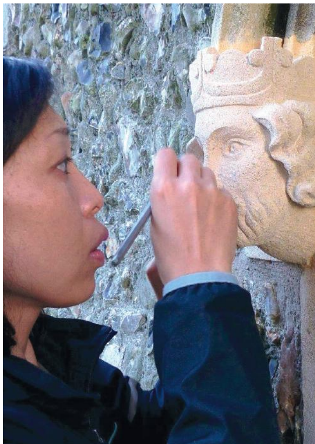
A stone mason carves a new figurehead at Willingale, St Christopher, as part of a large project to which The Friends contributed funds for roof repairs © David Kerwin
