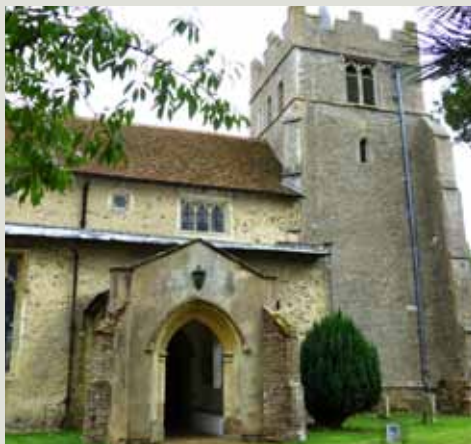
A grant of £4,000 helped All Saints, Ashdon make stonework and plaster repairs.
