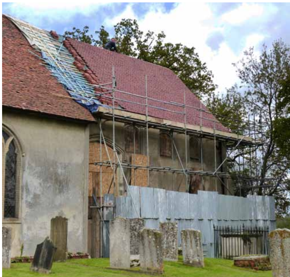
A grant of £15,000 to St Margaret's, Stanford Rivers in 2014 helped to get the church roof re-tiled last year.
